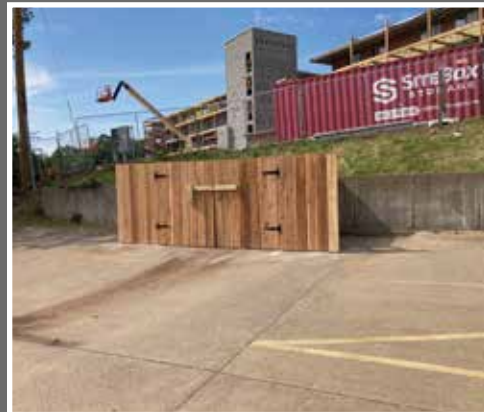
Completed reconstruction of the Trash Enclosure in parking lot. Royal Towers in background under construction, being converted into Condominiums.
